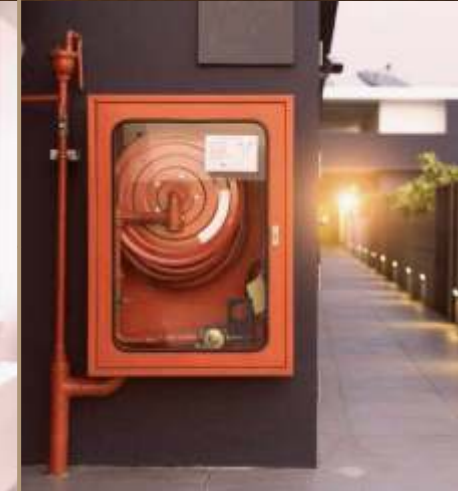
Fire Fighting System
